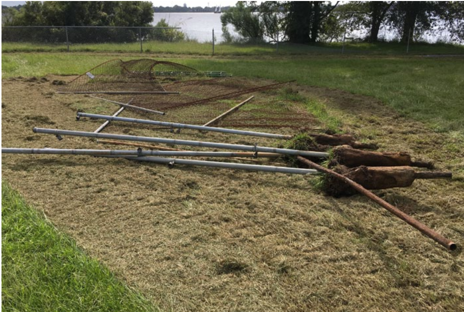
Remnants of the batting cage behind the old Bridgeton Elementary School ready for removal.
